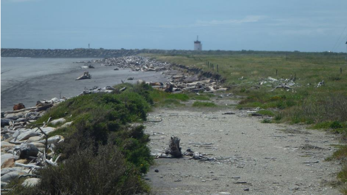
Figure 2-4: Erosion notch outflanking eastern end of airport revetment. Access from Rotary Road. [Credit: M. Hicks, 23/11/2016].
